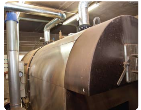
Wood-chip fired boiler at Wigram Lodge.
