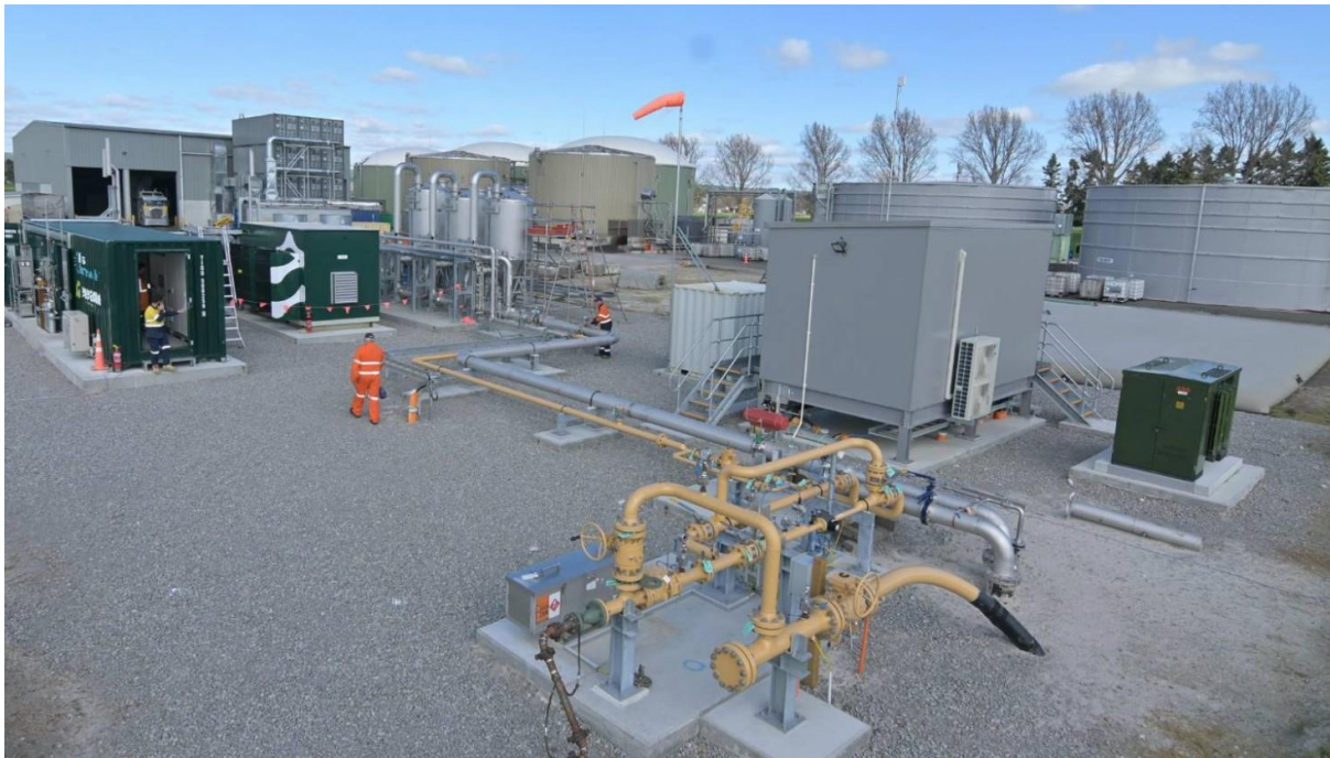
Photo caption: First Renewables Biogas to Pipeline Upgrade Facility at Ecogas' Organics processing facility in Reporoa.
