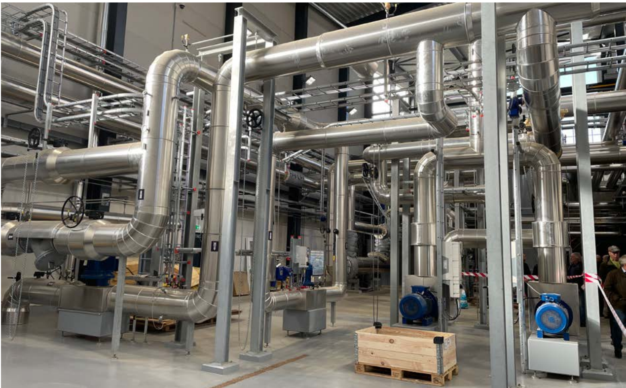
Typing at a district heating plant in Sorø (Denmark). The plant, operated by Sorø Fjernvarme, provides 12 MW of bioenergy to 1,600 customers based on the company's retrieval of garden and park waste (Source: Sorø Fjernvarme/Photo by AffaldPlus)
