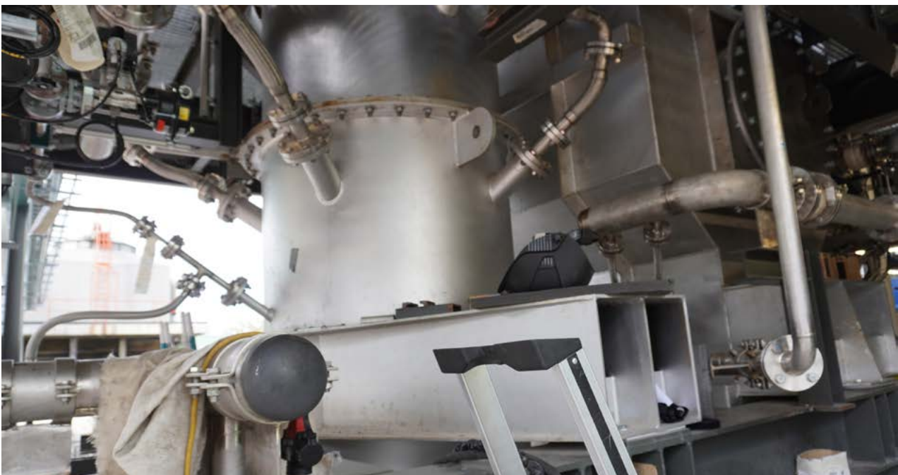
Combustion (front) and gasification (back) reactors in Vienna, with adapted reactor design to allow for the use of biogenic wastes (Photo credits: BEST)
