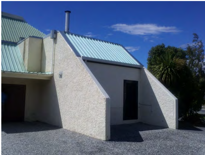
Figure 18.2 Pool site- LPG boiler (300kW- less than 10 years old ) located in ex-coal boiler house with easy access and bunker storage
