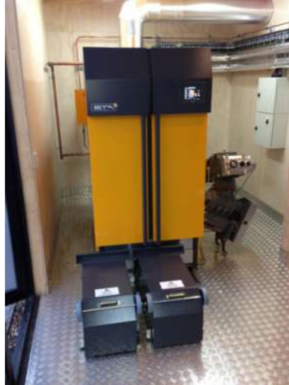
Spark Energy 200kW
