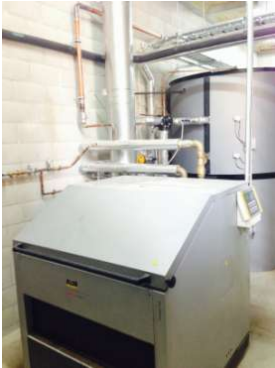
Aro Ha district heating
