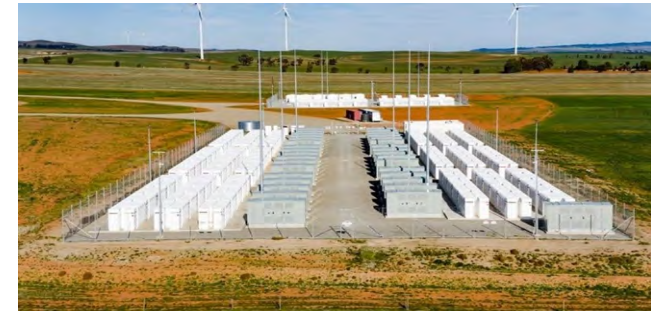
Figure 7: Hornsdale power reserve
