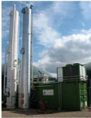
Catalyst Greenlane® Rimu – Fully Installed
